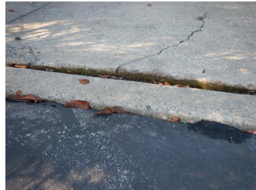
Large elevation shift between curb and walkway.
